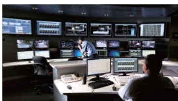
Command and control center
